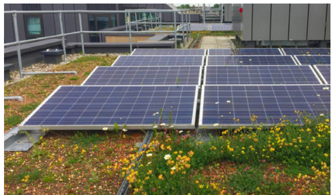
Biosolar roofs can reduce carbon footprint by minimizing heat gain and generating renewable energy.
