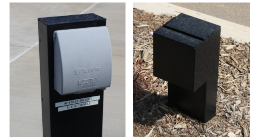
Example of a lockable power source and multiple power types, RTP HUB and Park Point (Source: Kimley-Horn)
